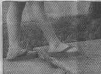
A tripping hazard should be called to the attention of the local government.
