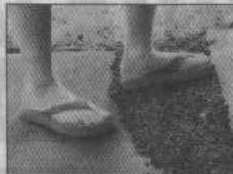
A temporary fix —in this case, old asphalt—minimizes hazard until permanent repairs can be made.
