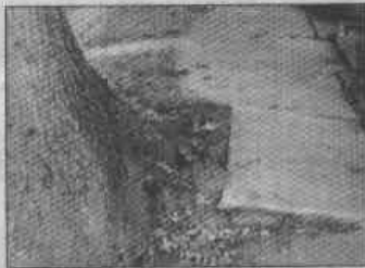
Tree roots are a major cause of sidewalk problems. Trees planted in the utility strip don't have room to grow.
