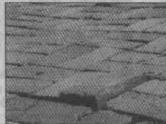
New brick is more hazardous than old because it is still settling and tends to get out of grade easily.
